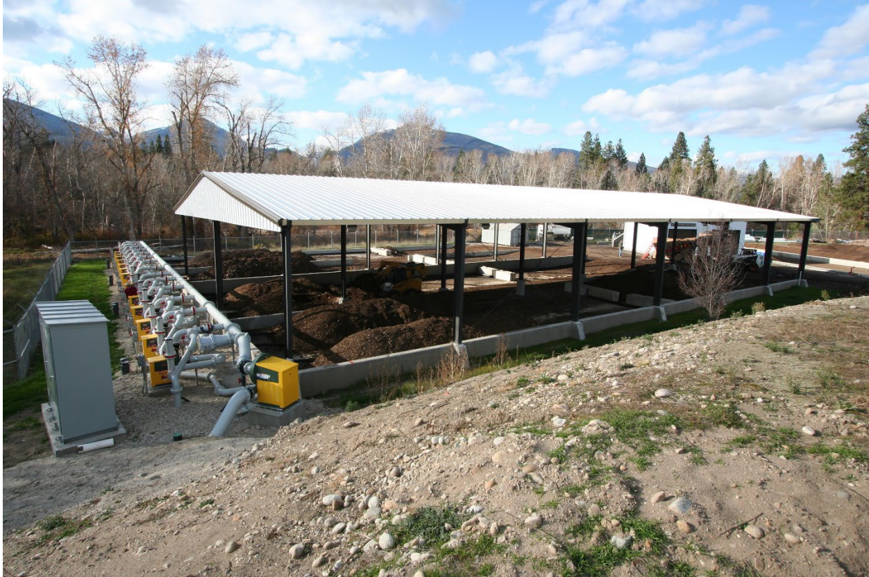
Figure 11. Hamilton, Montana Composting Facility
