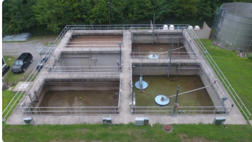
Figure 4. Example Exterior SBR Installation - Aqua Aerobic
