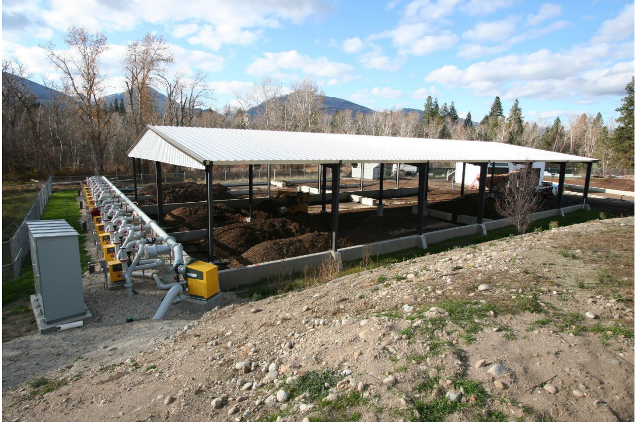
Figure 11. Hamilton, Montana Composting Facility
