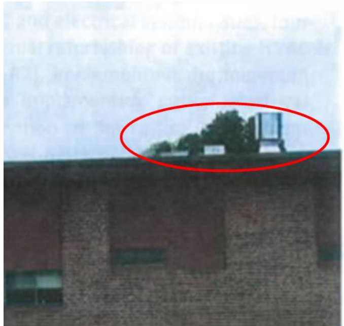
Figure 2 - Photo taken in 2013 of non-functioning heating and ventilation units on the roof of a Montana school.
