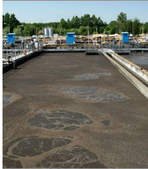
A wastewater plant with outside basins
